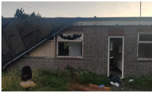
Photograph 1. Disused office buildings in poor state of repair.
